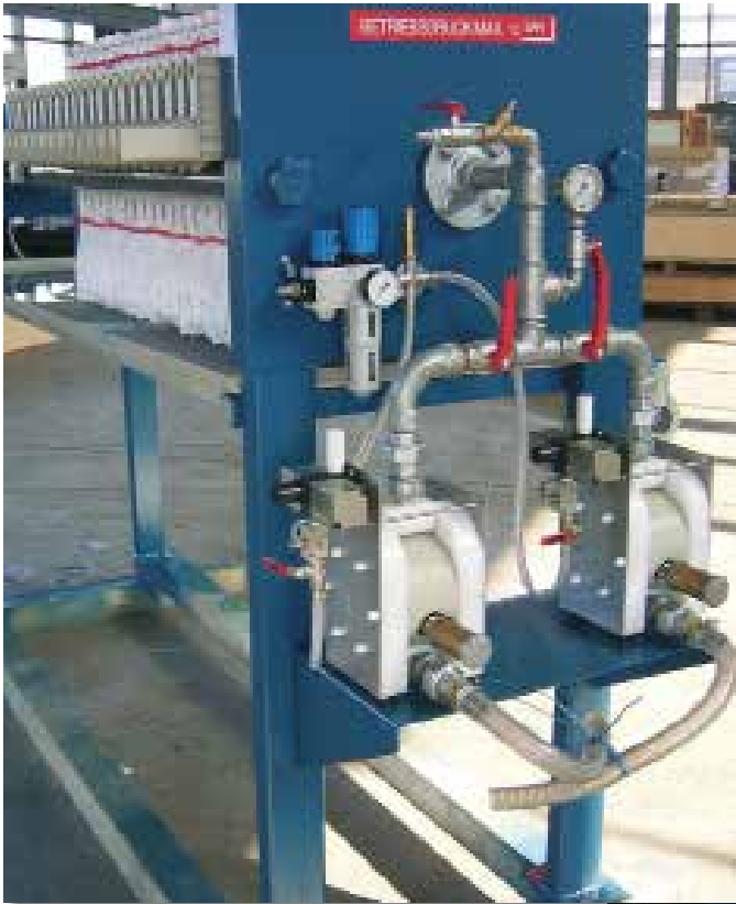
◀ Compact TF filterpress pumps installed for recovering solid waste from water
